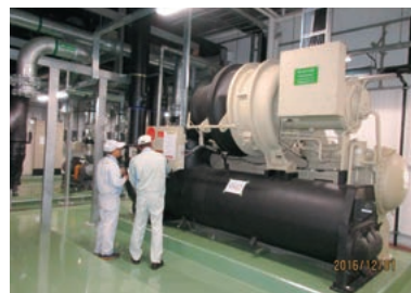
Turbo chillers installed at the Xicen Plant in China
