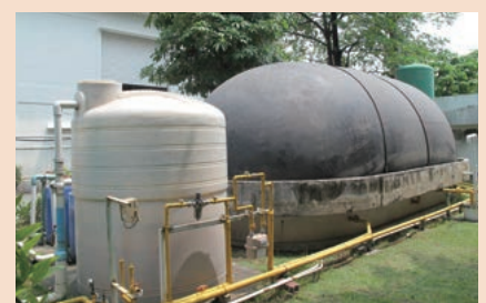
A storage tank for biogas
