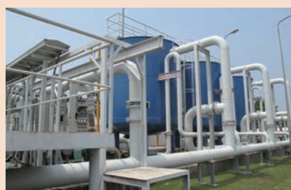
Facilities for a plant wastewater zero system
