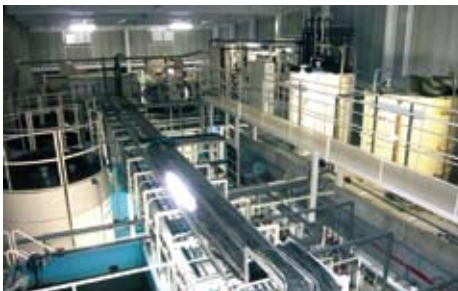
Wastewater treatment facility at the Fujisawa plant
