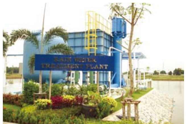
The rainwater recycling facility and reservoir at the plant in Bang Pa-in, Thailand
