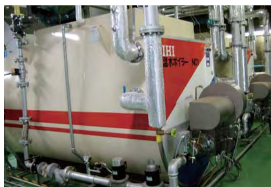
City gas boiler in Karuizawa Plant
