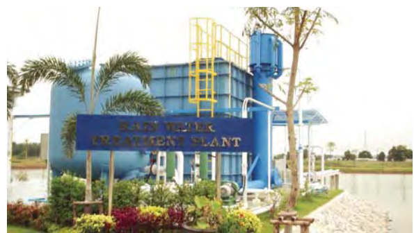
Rainwater treatment plant and water reservoir of Bang Pa-in Plant in Thailand
