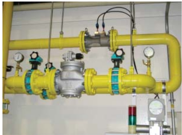
Compressed air flow meter and pressure-reduction valve
