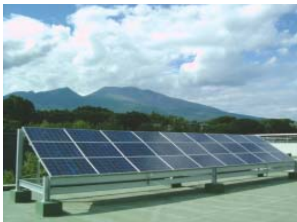
Photovoltaic panels at the Karuizawa Plant with Mt. Asama in the background
