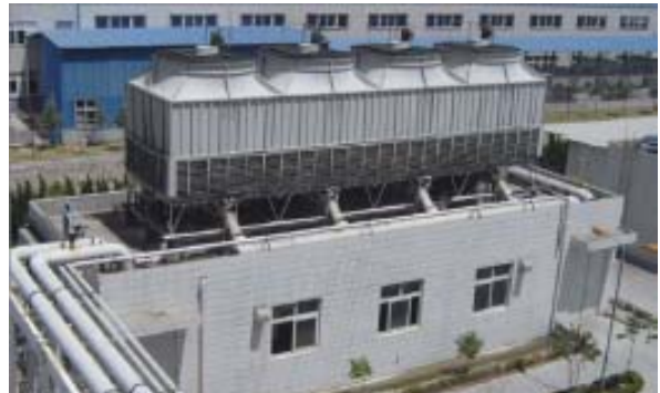
Shanghai Shunding Technologies' cooling tower
