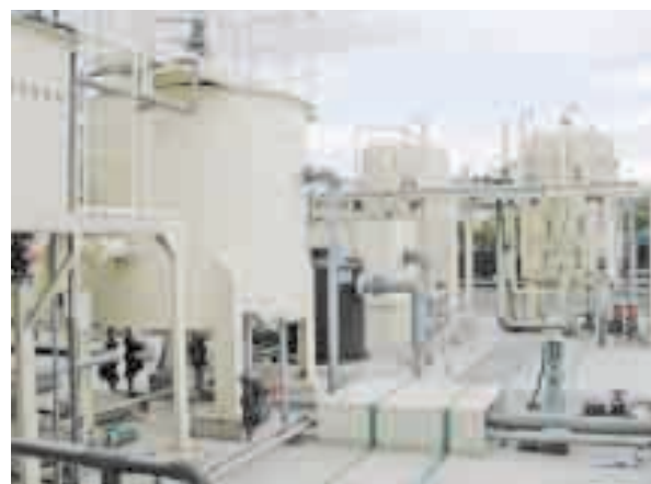
Wastewater treatment facility, Fujisawa Plant (Japan)
