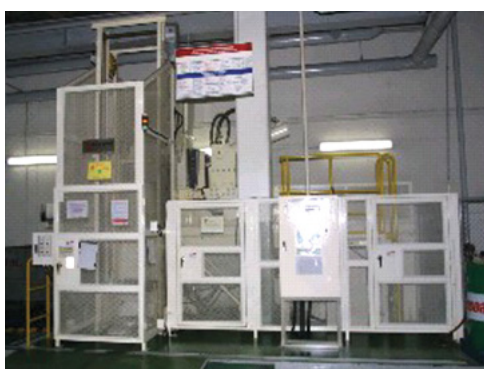
Oil recovery equipment
