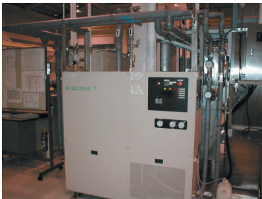
Exhaust recovery system installed at Karuizawa Manufacturing Unit
