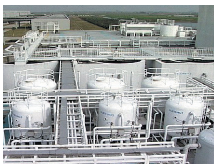
Wastewater processing facilities (Shanghai Factory)
