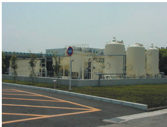
Wastewater processing facilities (Fujisawa Manufacturing Unit)
