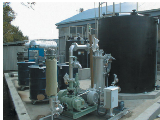
Soil and groundwater purification system at the Fujisawa Manufacturing Unit
