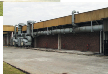
Oil mist collectors (after)
